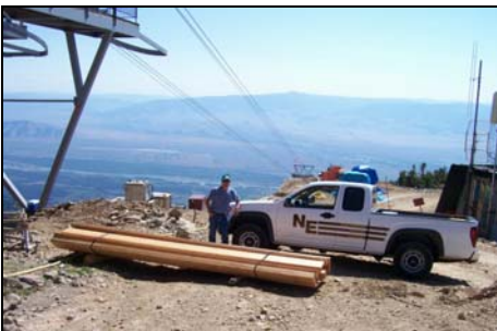
JACKSON HOLE SKI AREA AERIAL TRAM Teton Village, Wyoming
