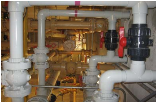
MEMBRANE BIOLOGICAL REACTOR (MBR) Alpine, Wyoming
