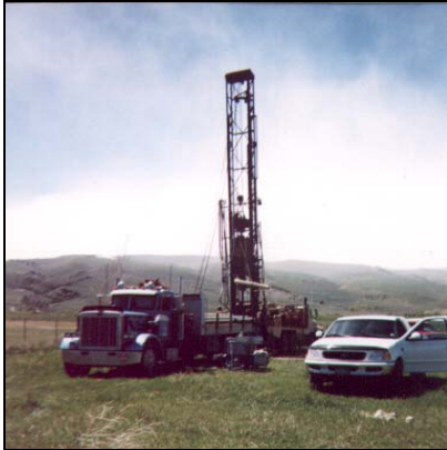
Aquifer Test Well No. 2 Lander, WY
