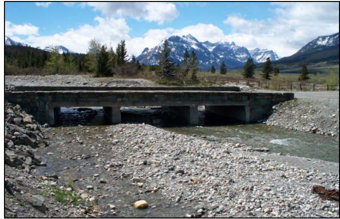
GLACIER NATIONAL PARK - DIVIDE CREEK Flood modeling and risk analysis for NPS facilities
